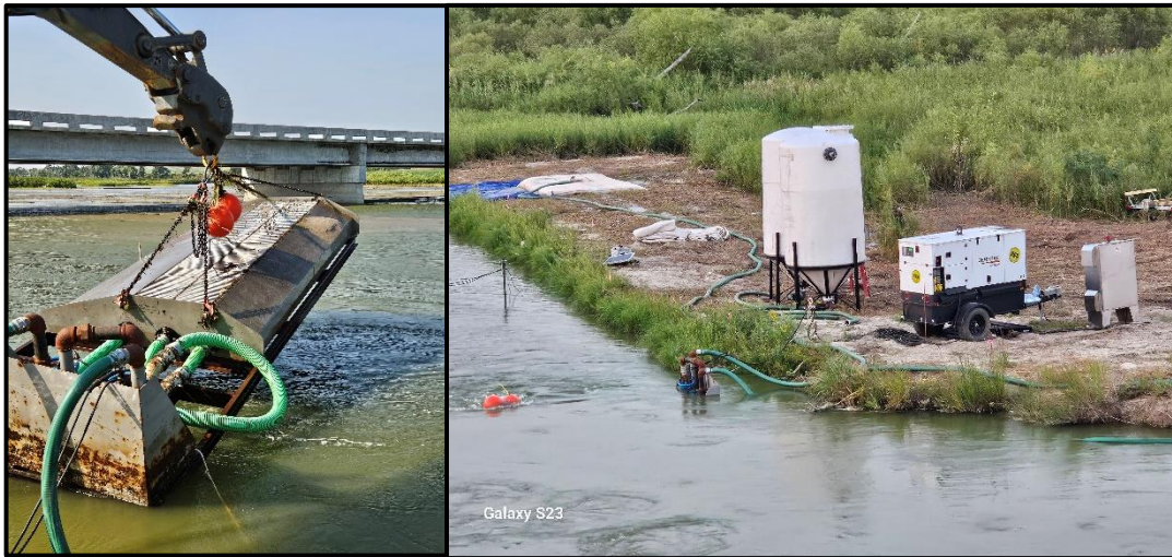
Figure 1. (Left): Niobrara River bedload sediment collector deployment. (Right): Site setup with generator, control box, collector in the river, sediment separation tanks, and dewatering tank to capture large volumes of sediment.
