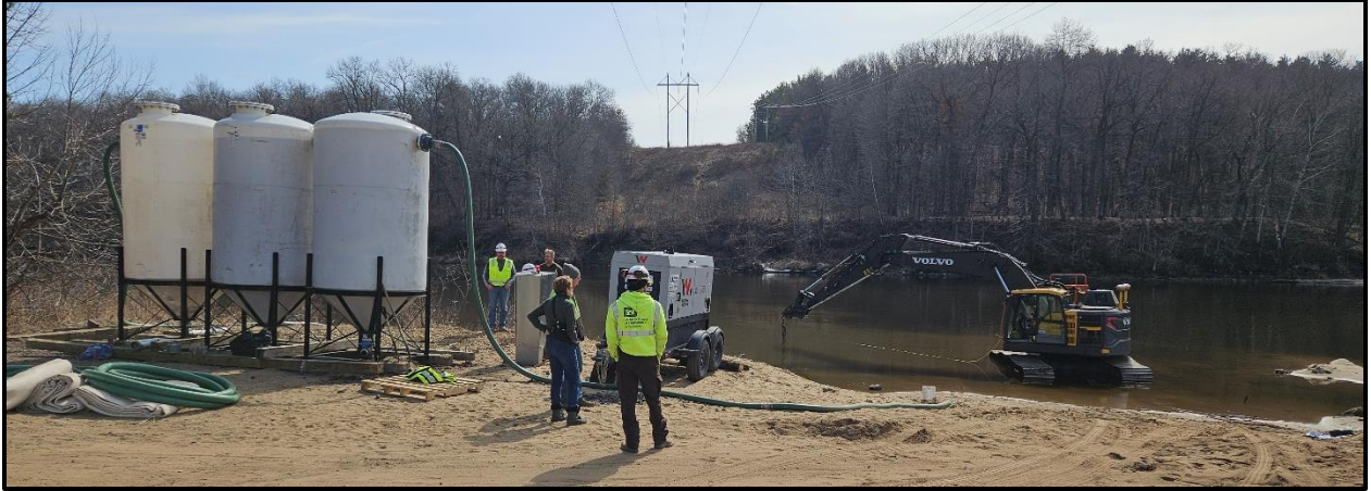
Figure 2. Bedload sediment collector site in the Eau Claire River, Wisconsin, 12 March 2024. The generator runs the pumps through a control panel. The large sediment separation tanks are for quantitative analysis to assess sediment collection rate for a given river flow, with the objective sampling the full anticipated range of flows.
