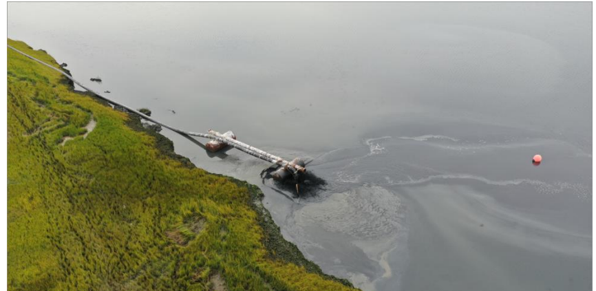
Figure 1. Placement of mud berm along the marsh edge at Gull Island, NJ
